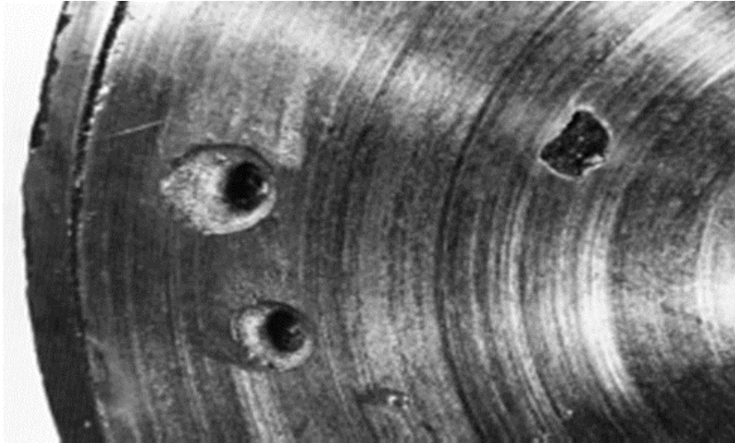
Figure 8. Pitting corrosion on the impeller (Cebeci, 2016).
